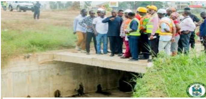
Work begins on underground drain at Kaneshie First Light to prevent constant flooding
